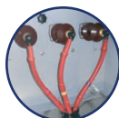
Cable Box for HV Bushing
